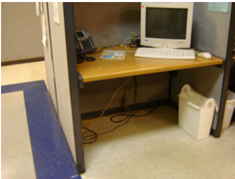
Cubicles with Poor Wire Management
